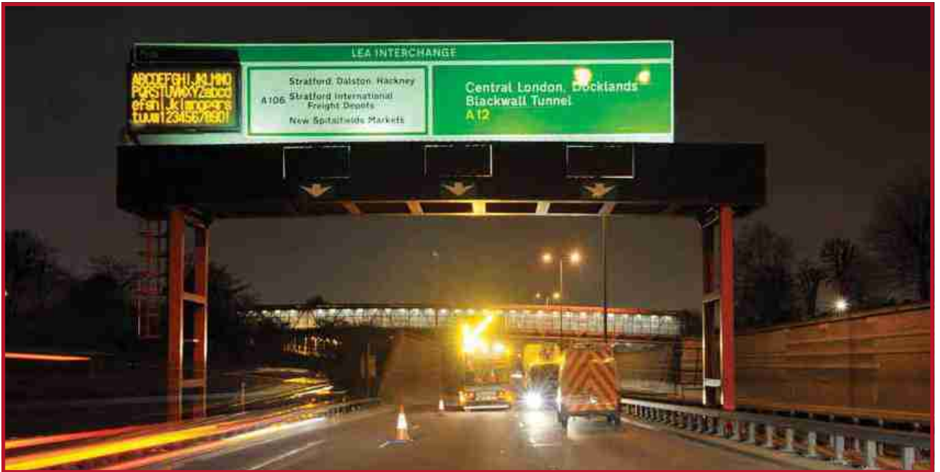
Large installations (recent signage project on the A12)
