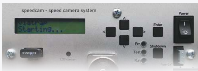
Control panel inside the battery box.
